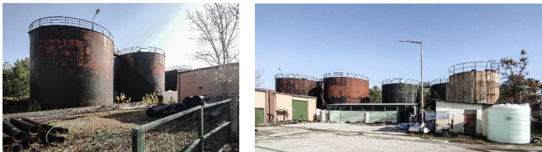
Figure 3.10. Central Heating Plant and Fuel-Oil Tanks, taken by the author
